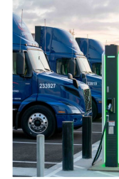
HD EV Charging Infrastructure
