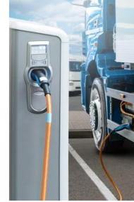
Heavy-Duty Electric Vehicle Charging Infrastructure
