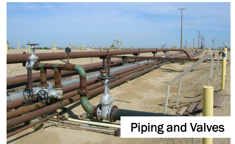
Sulfur Removal System
