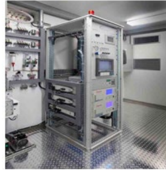
Continuous Emission Monitoring System (CEMS)
