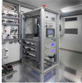
Continuous Emission Monitoring System (CEMS)
